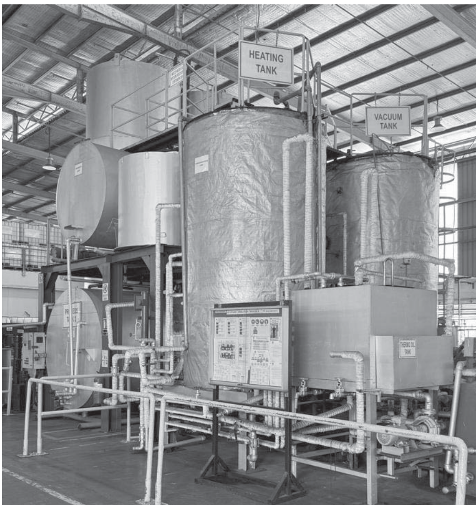
One of our waste oil recycling systems
