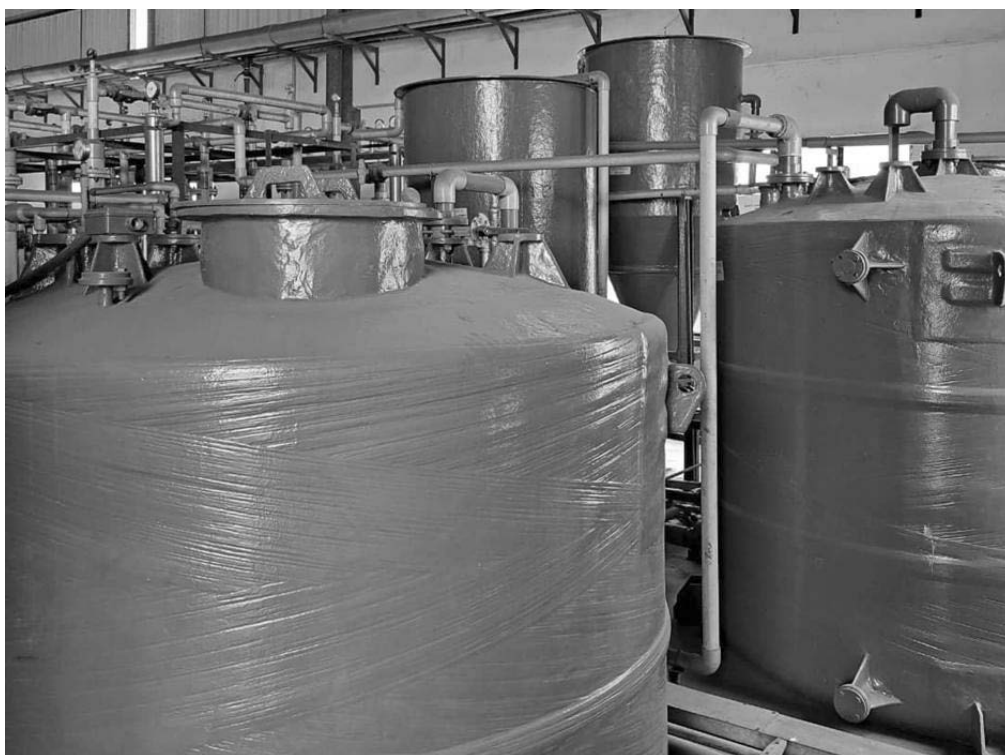
One of our waste acid recycling systems
